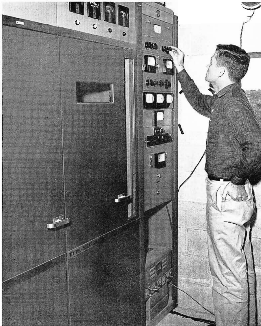
FIG. 16. View inside transmitter building showing engineer tuning speech rack (No. 3 rack). Cabinet No. 1 (extreme left) contains phasing equipment. Cabinet No. 2 is the BTA-500MX.
