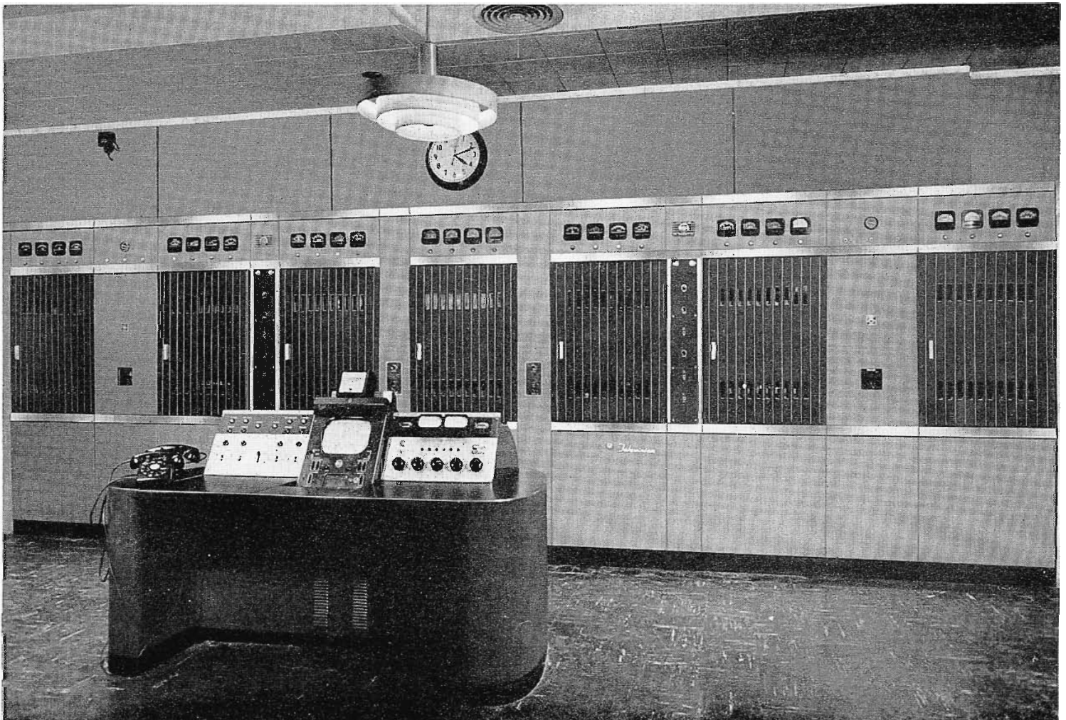
FIG. 9. The 25-kilowatt transmitter installation. No new cabinets have been added, however, spacing of the cabinets has been changed slightly to make room for the water columns.
